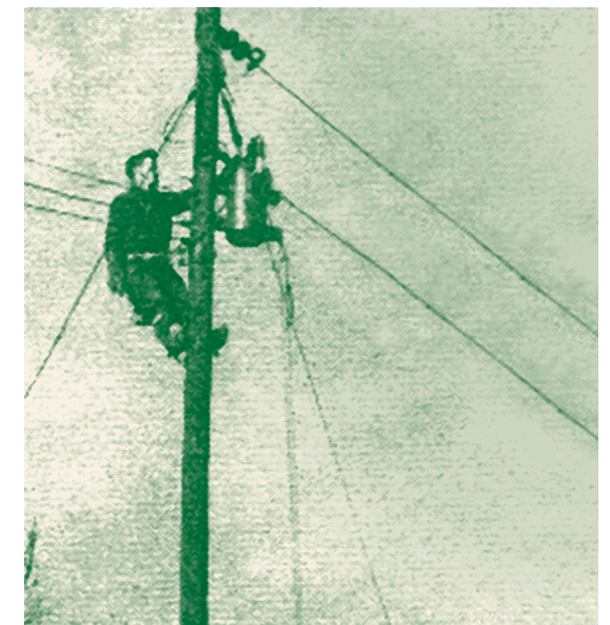
On January 15, 1940, the first GVEC lines were energized giving 150 Gonzales County farmers in the Bebe-Monthalia area electric energy for the first time. Just two months later at the first GVEC annual meeting, it was announced the Cooperative had built 225 miles of line and was serving 360 consumers.
