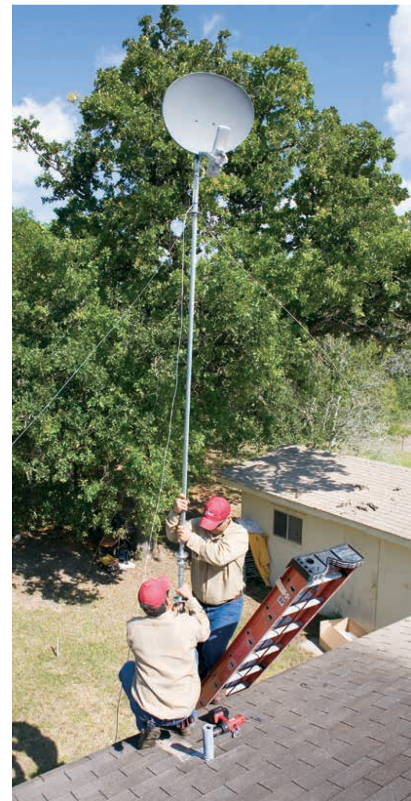
In 1998, GVEC.net was established initially offering dial-up Internet services, then moving into high-speed wireless technology. Crews and equipment were a welcome sight for customers as GVEC.net was the only Internet service provider in the rural area, and in many locations, remains so today.
