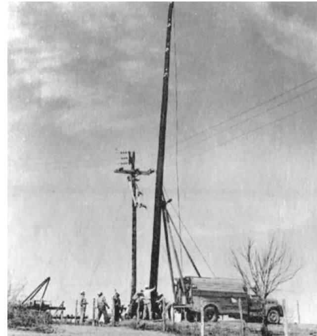
GVEC was among very few distribution cooperatives financially stable enough to construct its own transmission lines in the 1960s. Extra-long poles were required for the new 69,000 volt transmission line, which were a first for the GVEC line crews.
