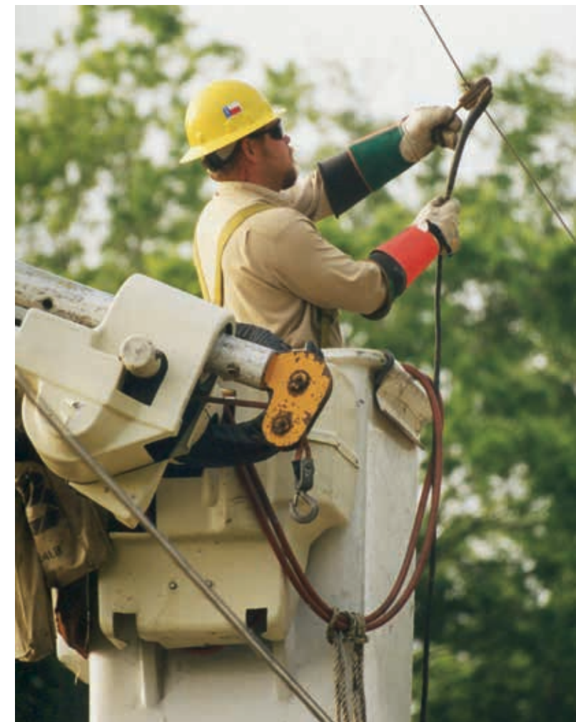
With ever-increasing voltages, one of the most important elements of safety in line work has been the evolution of personal protective equipment. Line workers such as Seguin Line Superintendent Keith Boenig, approach every project with the belief that "I am my brother's keeper"; a constant reminder that proper equipment and teamwork can and does save lives.
