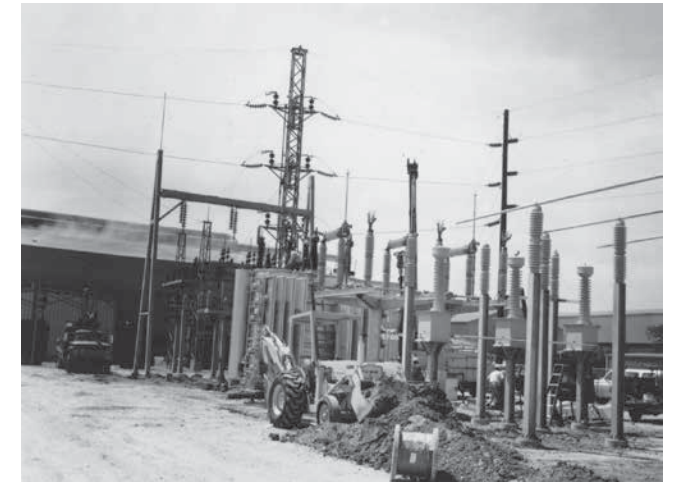
Construction on a new substation dedicated solely to the operations of Seguin’s steel mill, Structural Metals Incorporated (SMI), was in process in April 1975.
