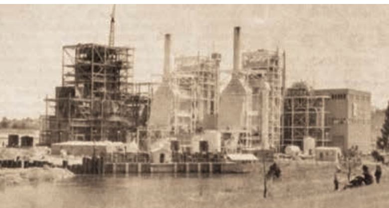
With demand exceeding more than hydropower could produce, LCRA built its first major steam electric generating plant, the Sim Gideon Steam Plant in Bastrop, shown here during the final stage of construction in 1965.
