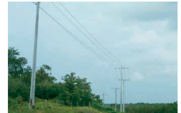
From 2011 to 2013, GVEC built five hundred miles of three-phase electric line and eight substations to serve the addition of approximately one thousand new commercial meters and hundreds of new residential meters stemming from the Eagle Ford Shale activity.
